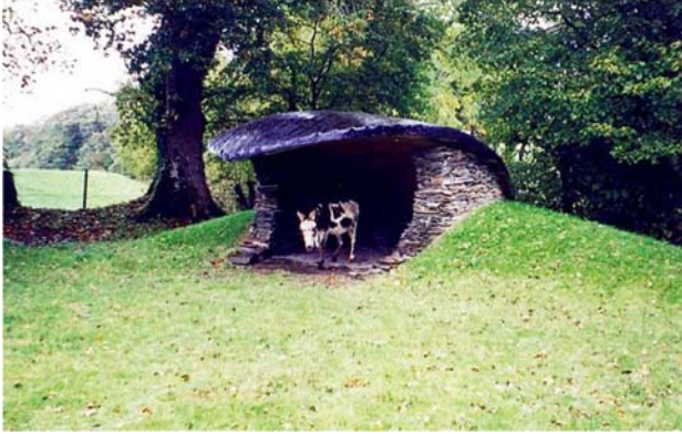
Figure 14 & 15. Figures 14 & 15. Tierney Haines Architects (2014) Construction of a simple shelter for two donkeys. The form takes inspiration from the impression of a donkey's hoof in the mud. The roof is made from canvas and tar over a bent wood frame in a similar fashion to west of Ireland curraghs. The stone is slate from the local disused slate quarry [Photograph] Accessed from http:// www.tierneyhaine.com
